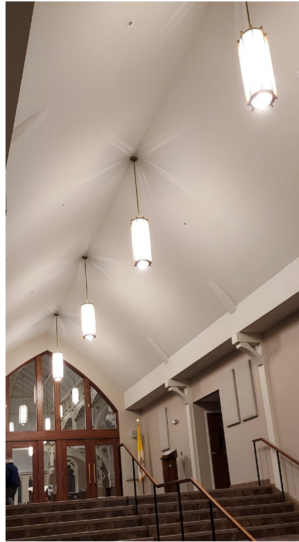
LED light fixtures
