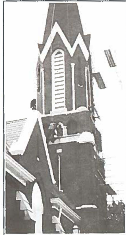
"You couldn't get me up there for BIG bucks!" one parishioner was heard to say. But "up there" is just where the workers went, painting the wood trim, caulking the windows, sealing the brick against damage from rain and sleet and snow. And now St. Patrick's church is snug and fit for several more years of community worship in prayer and song.
