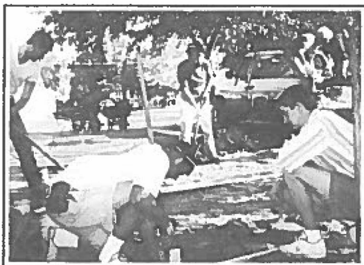
Men from the Building and Grounds Committee and the Urbana Knights of Columbus gathered early on Saturday, October 1, to lay a foundation for the patio area on the east side of the church. Volunteers, captained by Steve Marsh, included Mark Nirider, Chris Stohr, Ray Alane, Jim Mayer, Mark Simon, Chuck Shaw, Walt Mikolaitis, Oscar Kocher, Terry Bosley, Jim Risatti, Tom Kacich, and Bill Van Cleave.
