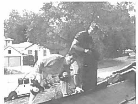
With its new roof, the Kirks' home will be snug and dry this winter, compliments of St. Patrick's volunteers. Chuck Shaw (left) and Arden Howey were two of the many who came to help
