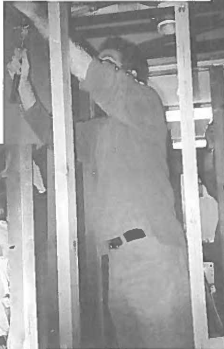
Andy Stumpf is determined to remove every last bit of plasterboard up there.
