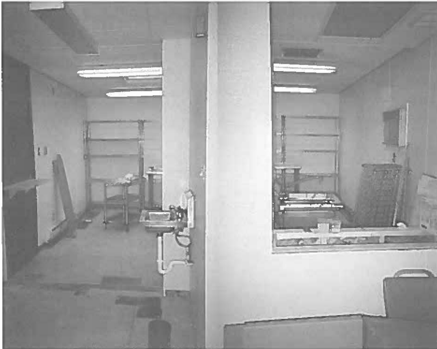
Nearing completion, the food pantry would be in operation just a few days later!
