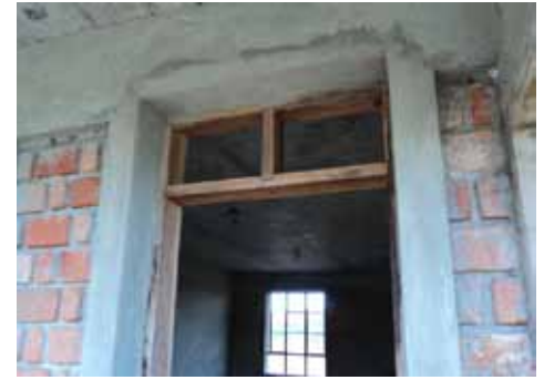
Close-up of an entry to one of the school buildings—all made through the efforts of local people without the benefit of construction equipment.
