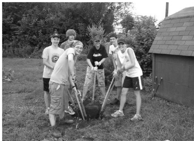
Mary, Dan, Josh, Julia, Will, and Kaitlin dig out a very big cement fence post!
