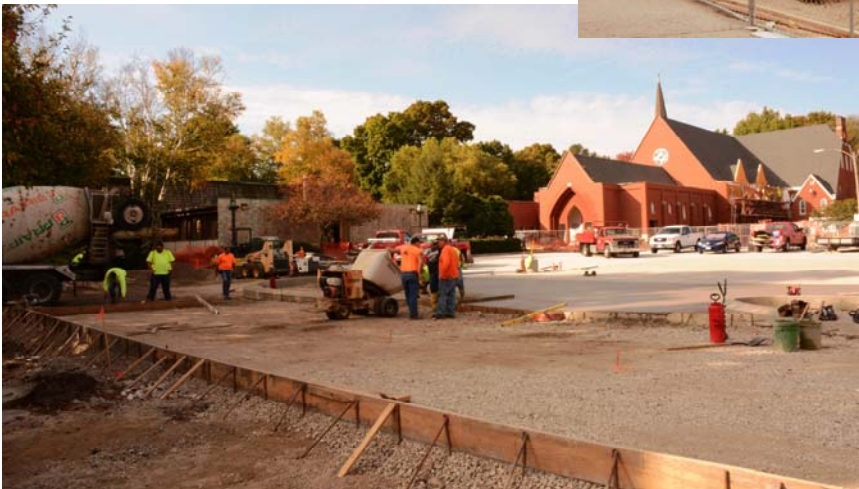
New parking lot construction with view of new addition This photo of concrete being poured for the new parking lot also provides a great view of the new addition.
