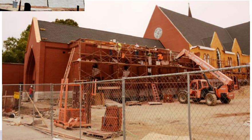
North side view of the church from parking lot Work crews complete the first section of bricking on the north side of the new addition.
