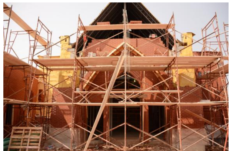
Exterior view of new east entrance Through the scaffolding, new brickwork and arches appear, giving shape to an attractive and welcoming new entry.
