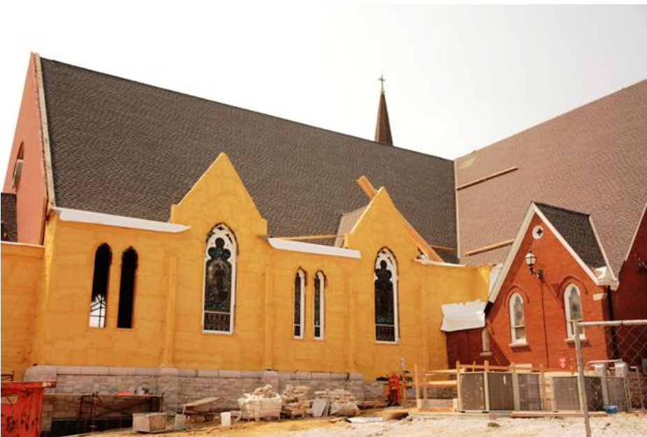
Exterior view of stained glass window, north side Progress continues as the stained glass windows are installed in the new addition—a wonderful blend of the old and the new!
