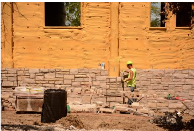
Exterior view of construction, south side Stonework matching that of the old church gives our new addition the same traditional, classic look.
