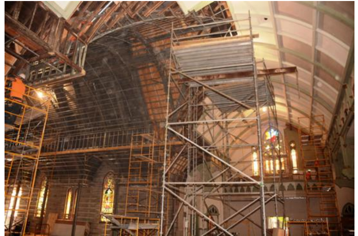
Interior view of connection between the church and the new addition, from the south
